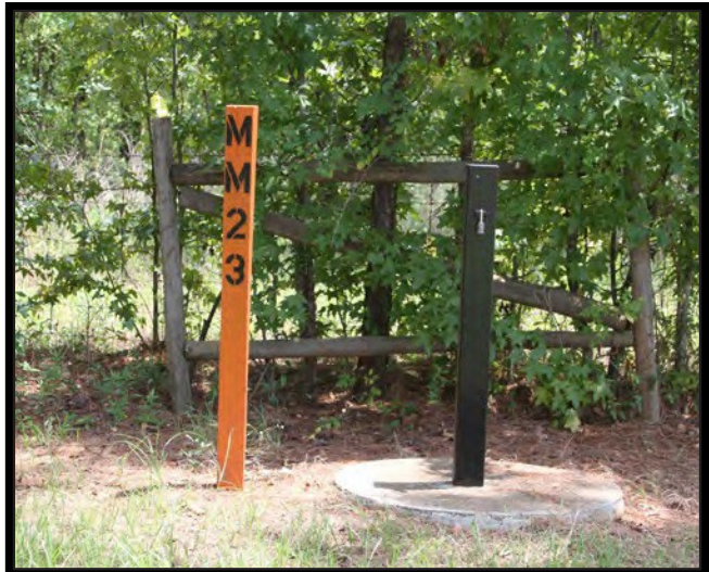
Methane Monitoring Well
