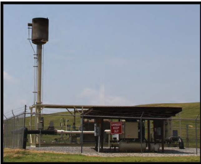
Methane Flare Station
